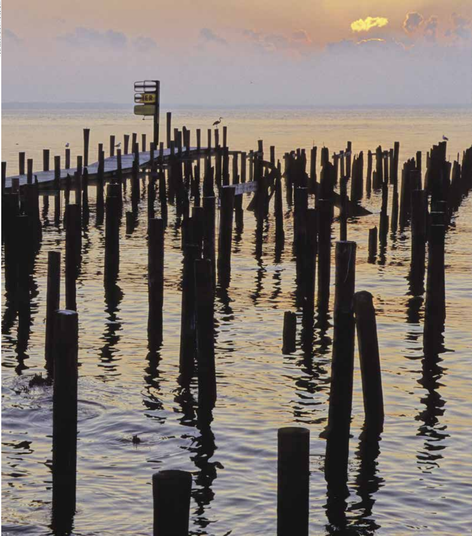
A pier that was destroyed in Colonial Beach, Virginia, in Hurricane Isabel on September 16, 2003.
