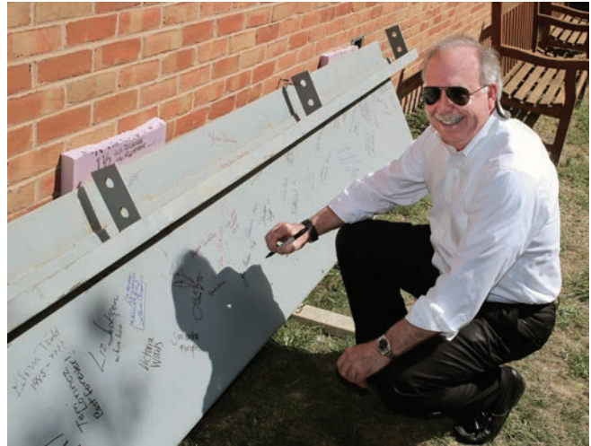
James A. Hixon J.D. '79, M.L.T. '80 joined members of the Law School community in August to sign the final steel girder for the Center before it was hoisted into place.
